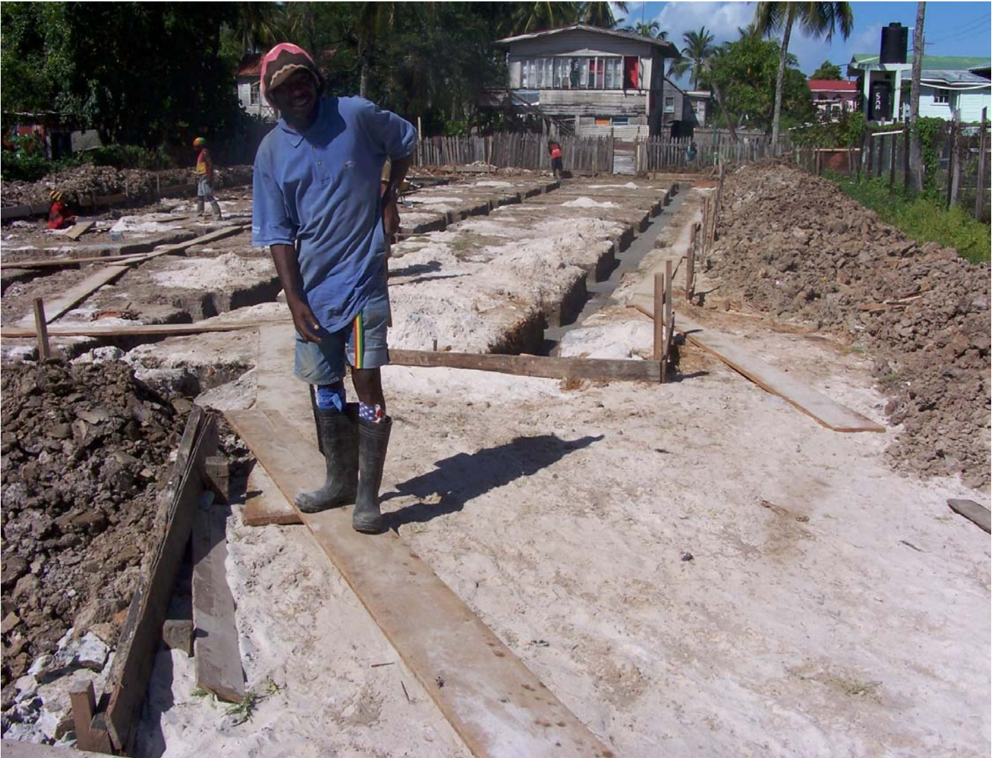
This picture taken on 13 th January, 2011 shows workers laying the foundation for the two-storey structure
